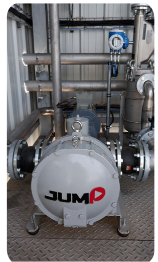
Pumping unit JE24s
